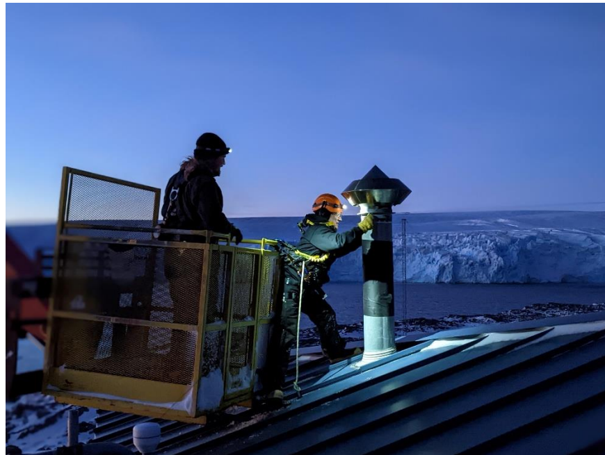
Carpenter and Antenna Rigger repairing the RASA ductwork. Image credit: Ben Rosen-Filardo.
